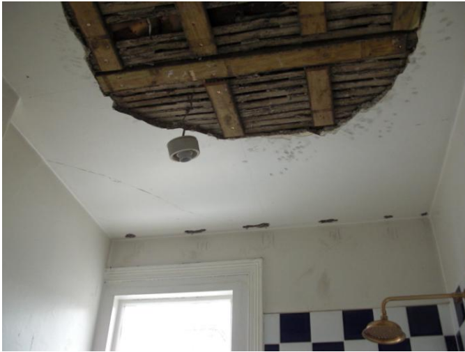
Before: Collapsed ceiling
